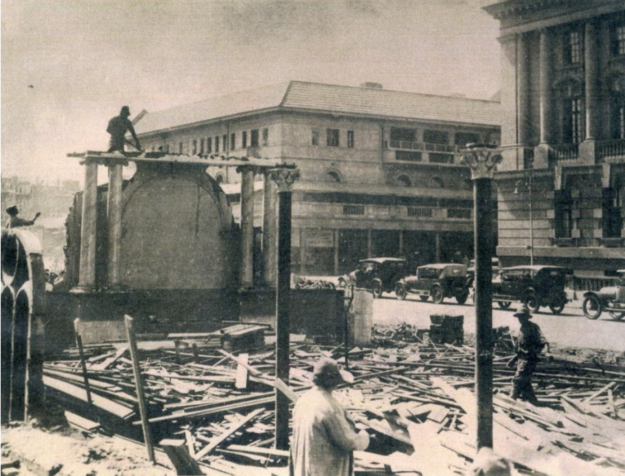
Photograph showing demolition in 1932 of a nearby building to make way for the new station. Old Park Station was retained as a functional platform. Museum Africa collection.
