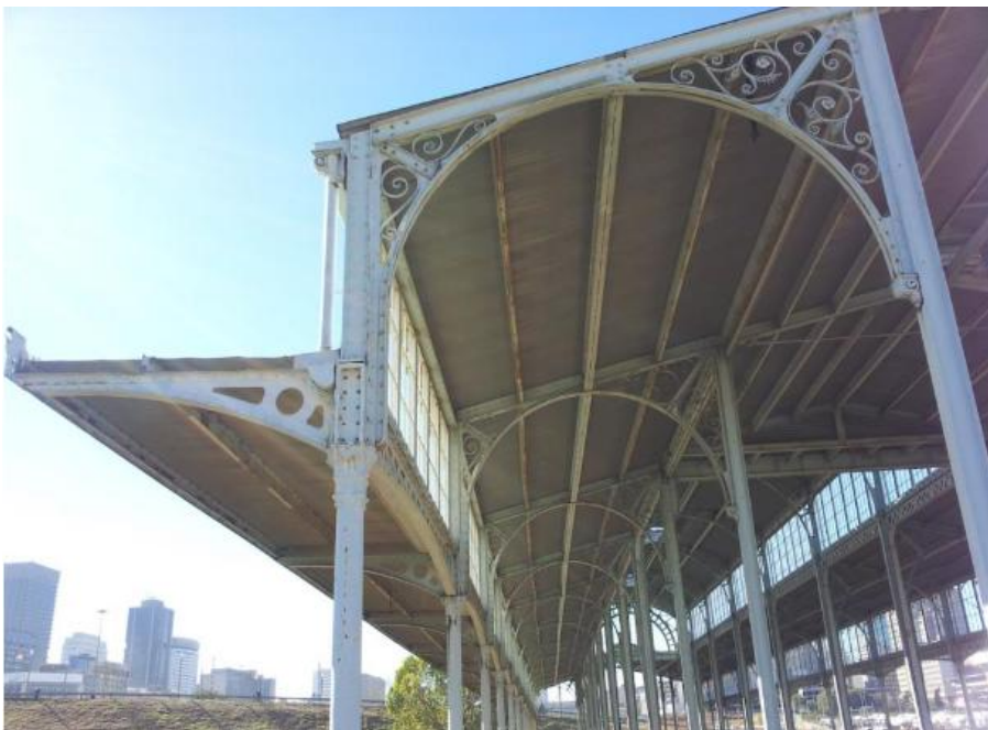
Photograph from 2013 showing the detailing of the cast iron structure and wrought iron ornament to Park Station, heritageportal.co.za
