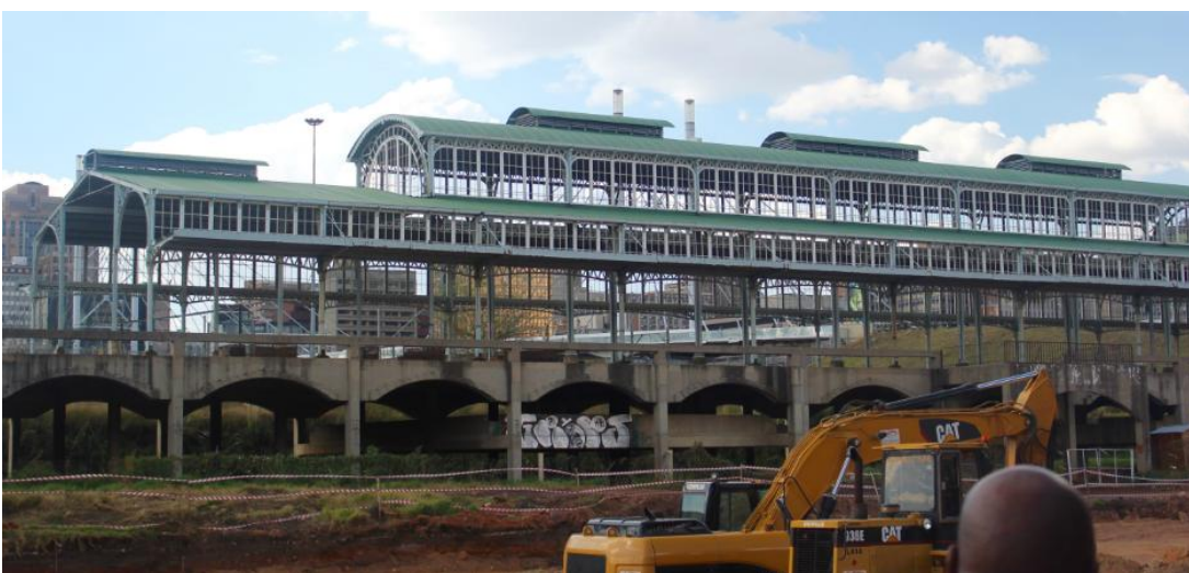
Photograph by Elodie Hazard for Johannesburg Heritage Foundation, April 2015, showing the cast iron and glass structure on the concrete podium, with site preparation work underway in the foreground
